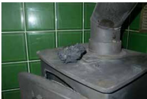
One of two, blocking the flue
